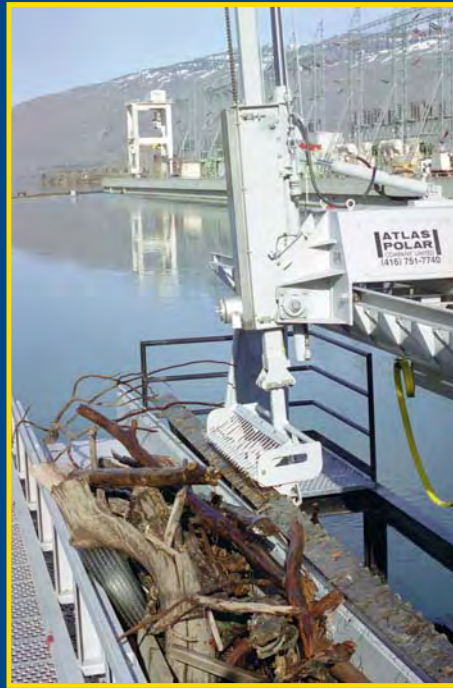
The popular Atlas Polar Hydrorake Trashraking System handles its job quickly and automatically raking trash from water intakes.
