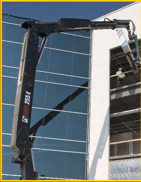
Delivering building materials further and higher with a long reach HIAB articulated crane.
