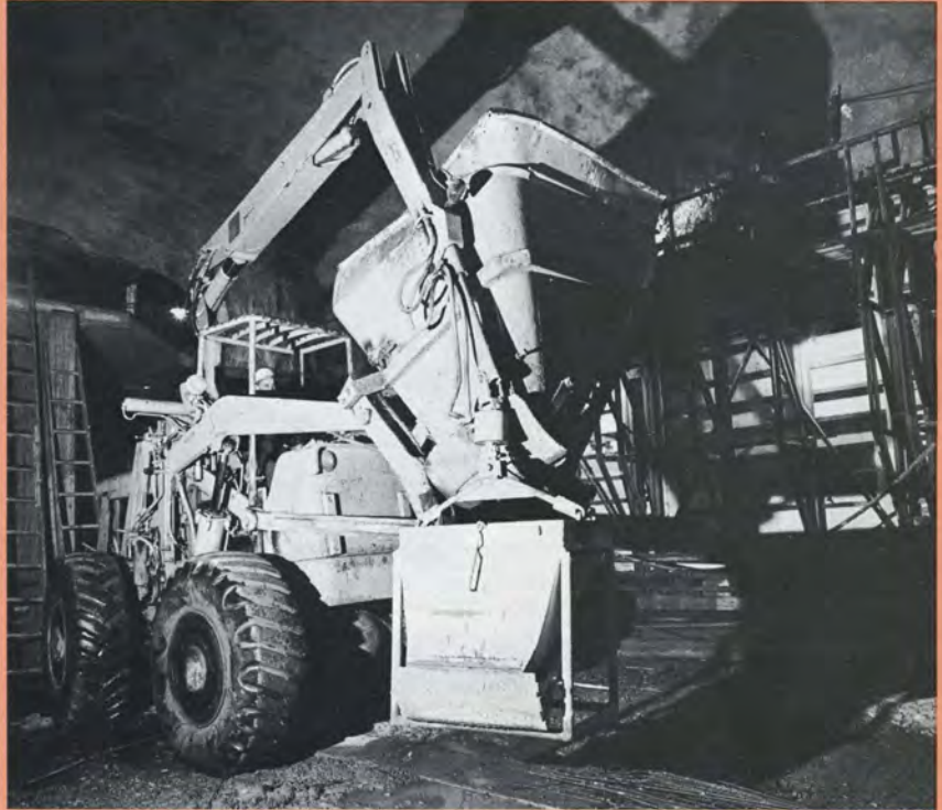
The skip is filled with concrete from Hilda's bin and is then hoisted by the crane and emptied straight into the form. (Another picture is on the back cover.) The bottom hatch of the concrete bin is operated hydraulically by the driver. The 3\frac{1}{4} yards held by the bin can be poured in ten or twelve minutes.
