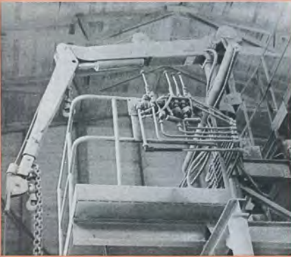
The intermediate crusher also has its HIAB crane, a 293, which is used for servicing work on the machine. Since the crane is on a high mounting it is equipped with a winch.
