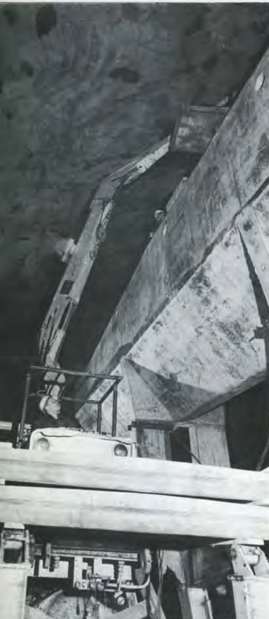
One of Hugo's important jobs is handling the concrete slabs that form the cover of the vent ducts. Screwed sockets are embedded in the slabs at the time of casting. When the slabs are to be lifted, eye-bolts are screwed into these sockets, providing points of attachment for the crane ropes. Thanks to his rotator, Hugo can then hoist the slabs—which weigh around a ton apiece—and deposit them in position with the millimetric precision that the job calls for.
