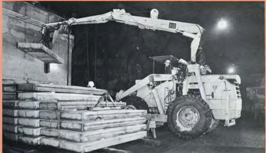
The concrete slabs for the covers of the vent ducts are cast at an underground concrete station. Hugo both loads the slabs and transports them to the site, piled on the fork of the machine.
