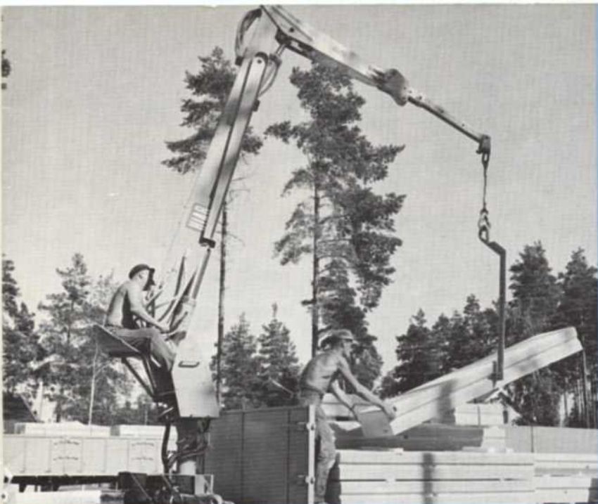
Clearly shown in this picture is the specially designed lifting hook, inserted in the hole near the middle of the unit. With the lifting force thus applied close to the C. G. the man on the truck deck need only steady the unit at one end to prevent it from suffering damage by striking against the truck flaps or against other units.
