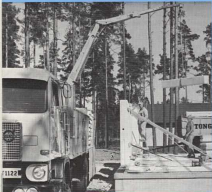
The lifting hook is replaced by a soft sling for handling the window lintels.
