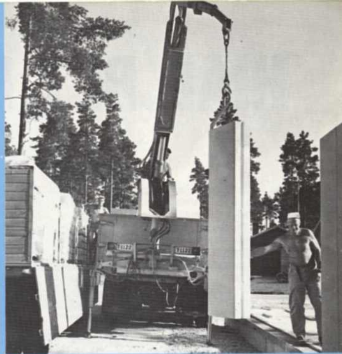
The wall unit is here being swung across to the foundation and tongued into the preceding unit to form an impervious wall. With the rear-mounted crane it is just as easy to lift the units off the trailer as off the tractor truck.
