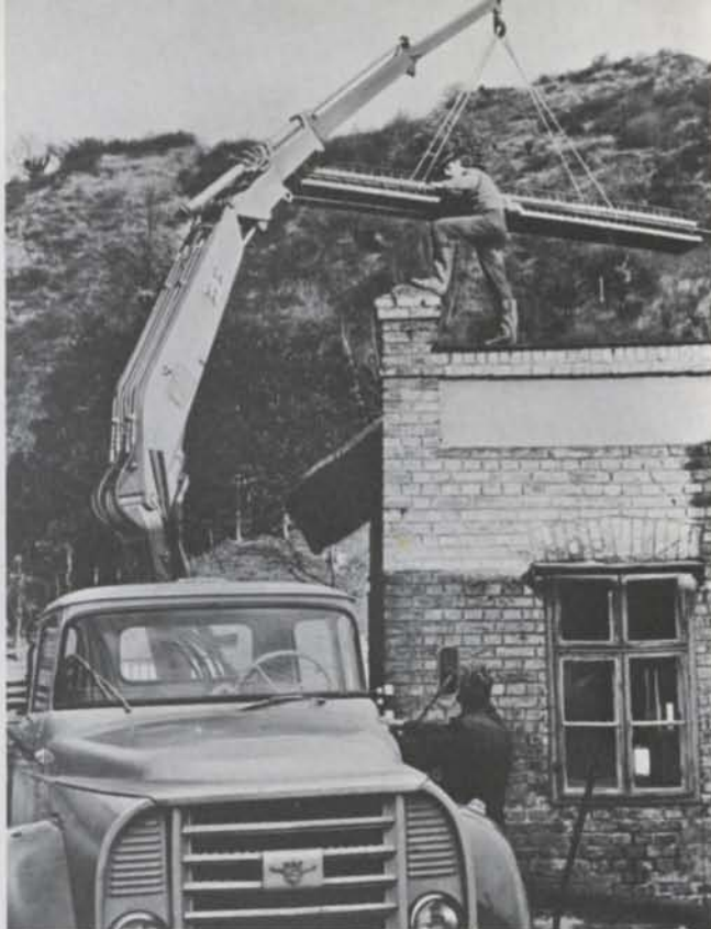
An extra jib section and the hydraulic extension gives this HIAB 174 Speedloader a lifting height of up to 36 feet—enough to put the roof on taller buildings than this one in Austria.
