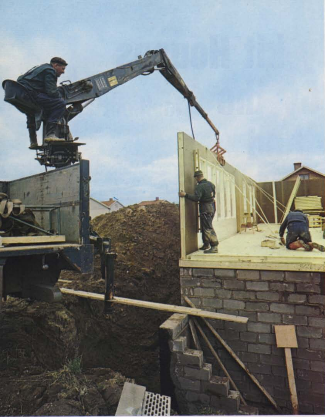
◀ The HIAB 177 Speedloader's first job is to lay down the floor blocks, and then, after hoisting in some interior fittings, it plants the walls straight into position. Since the blocks are to be handled by the HIAB Method they can be made large, and all the walls are erected within an hour or so.
