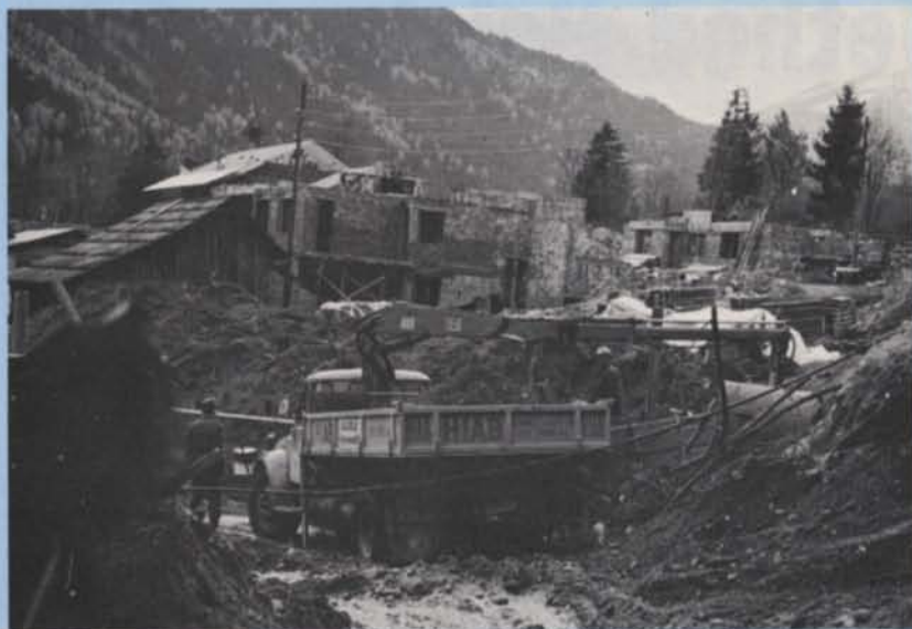
The HIAB outfit performed an important role in the building operations that were hastily started to house the victims of the disaster.
