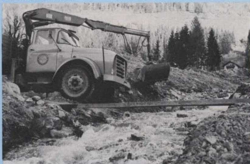
One of the first tasks assigned to the HIAB outfit was to clear away soil and mud swept down by the floodwaters.
