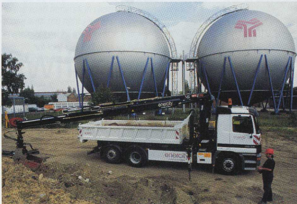
Filling material that may be needed for refilling is kept in intermediate storage. During his breaks, Reinhard Seybold collects any surplus and drives it to the tip.
