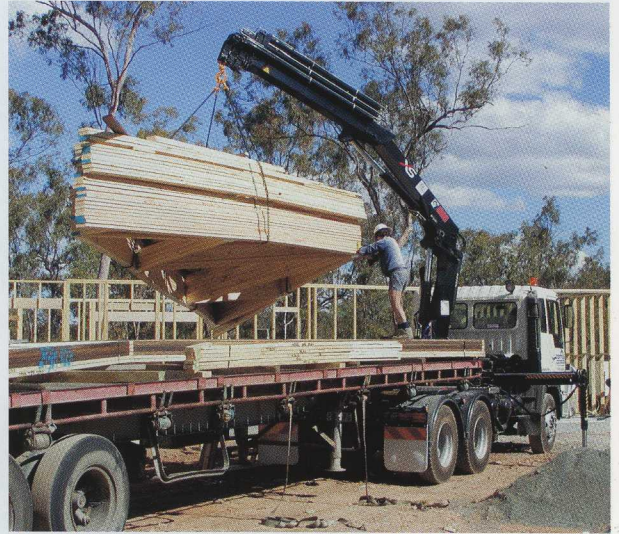
Nortruss exceed their customers expectations every day, with the help of their new HIAB XS 166 E-5 HiPro.
