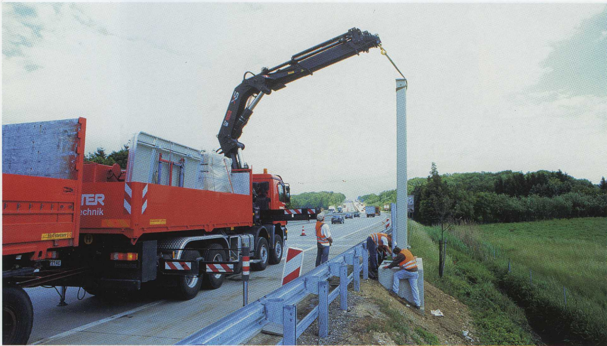
Forster signposting tasks are carried out by a well-functioning team. Here Harald Harreiter is operating his HIAB XS 700-8. To help raise and precisely position posts on newly cast foundations.
