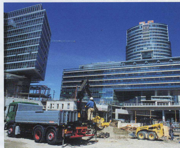
Paul Lachmayer appreciates the precision of the HIAB XS 122 E-3. He does not always have this much space to move around in as here, outside the Vienna International Centre and the new United Nation’s conference centre.
