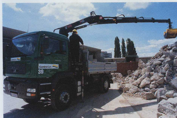
A HIAB XS 122 ES-3 Pro with clamshell bucket and rotator on a two-axle vehicle is a typical combination at ContraCon.
