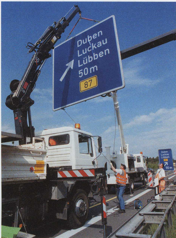
Signs to be erected and signs to be dismantled. An extensive improvement to the road network in Germany is generating a great deal of work and those with the right gear get the work. VTEAM work out early and invested in an XS HiPro – the first such crane in Germany.
