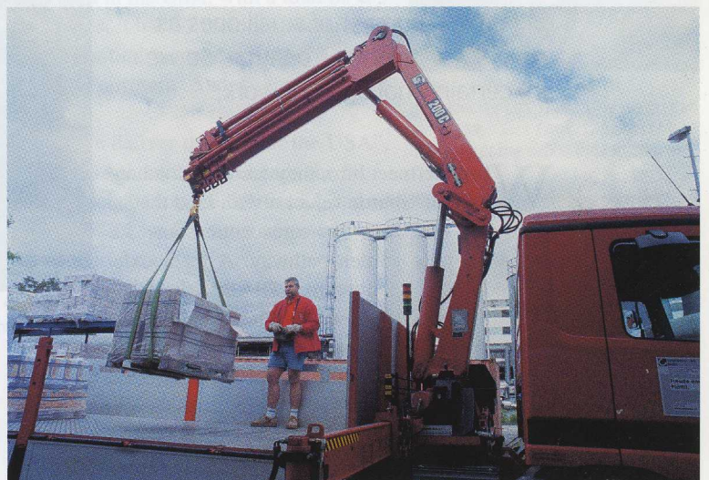
Patrice Scholler and Christofoli’s red truck with its red HIAB 200 C-5 crane is a familiar sight at building sites throughout Switzerland.
