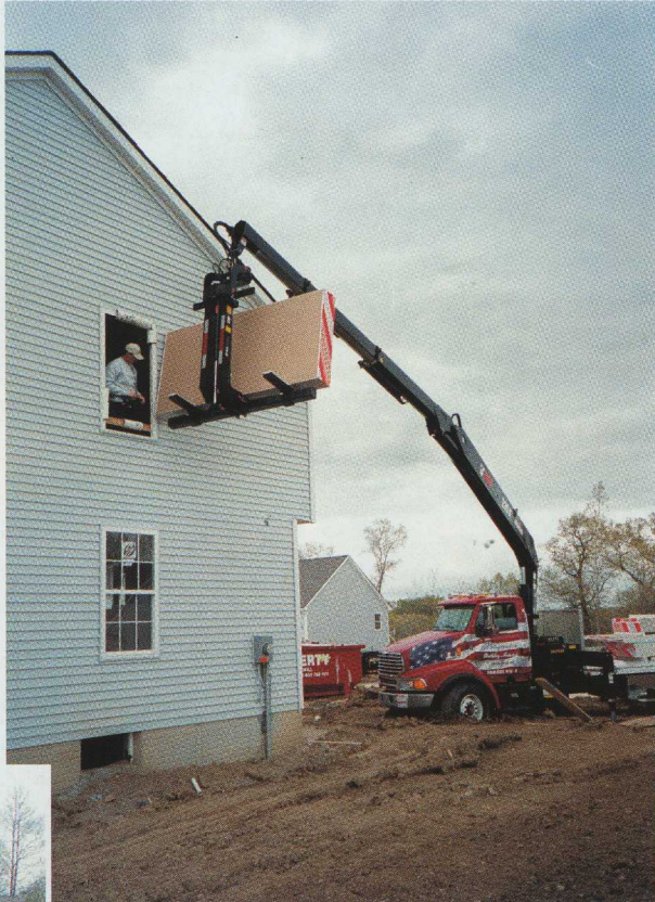
The HIAB 235 K offers all you need for precision jobs. Joe McCoy placed the cargo right outside the window and then all he and Jerry Brockway had to do was to start pulling in the plasterboard panels. As the pallet fork empties, Joe is able to adjust everything.
