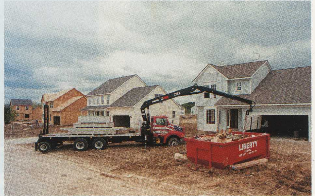
No fork lift would have been able to handle conditions here. A muddy site and a skip taking up the entire garage approach limited everyone's movements – save for the HIAB 235 K, that is.
