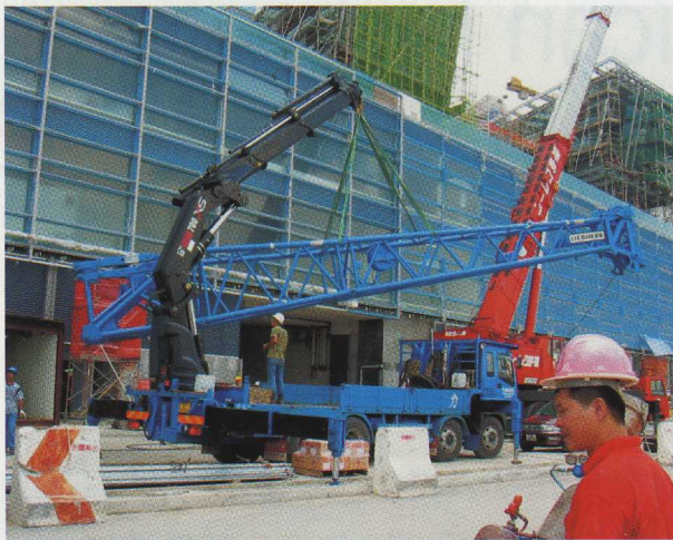
A HIAB XS 700 is used to assemble the big construction cranes. This one is being put together on the site of the projected 88 storey International Financial Centre.
