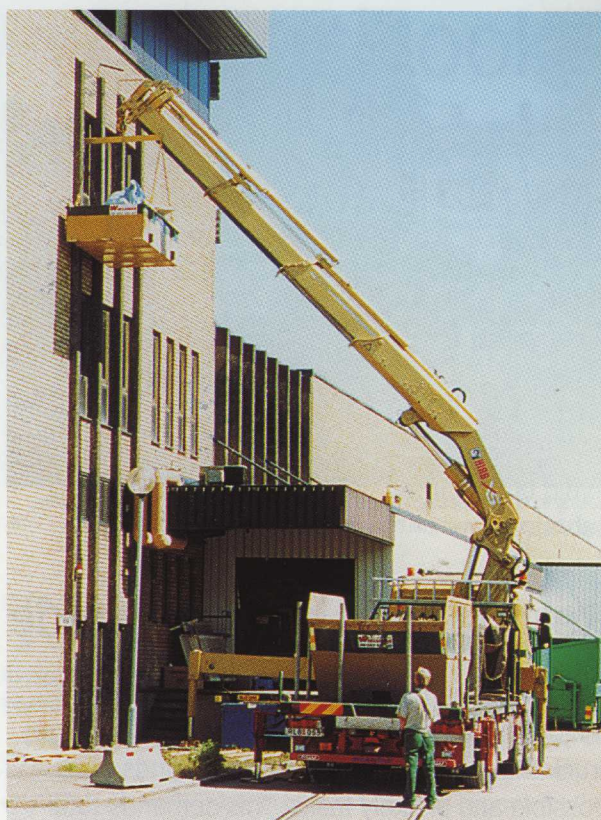
"The XS responds beautifully..." says Ove Lundell as he carefully places the container against the side of the building to help carry away the leftovers after a renovation job.
