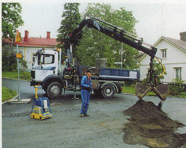
Calling in Reijo Seppänen saves a lot of time and labour. In the picture, Reijo is raising street gullies in no time at all using his XS 166 DUO.
