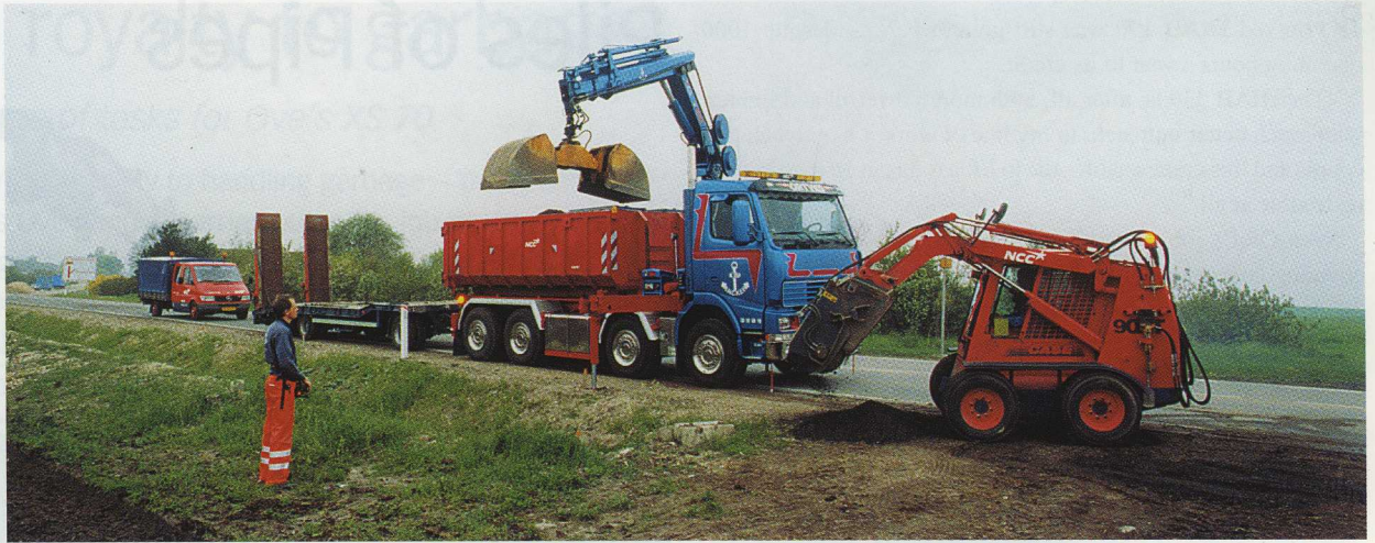
The road out to the ferry station at Sjællands Odde has had a provisional road surface during its "running in" period. Kim Ancker is removing this to get rid of the unevenness when the permanent surface course is laid. He loads the truck with the help of the bucket while the old asphalt is removed and put in a pile.
