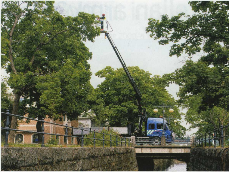
The personnel basket is in regular use. "I can reach up about 20 metres and the working radius is 30 metres. It is very practical as this means I don't need to move the truck so often."
