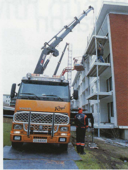
Tom R. Oppegaard can extend his crane to a maximum of 24 metres with the help of the HIAB 245 E's seven hydraulic and two manual extensions. That gives him plenty of margin to lift the roughly 400 kilogram heavy balcony units into place on the 4th floor.
