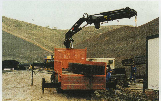
To make the intensive contacts between Madrid and Barcelona easier, a new high-speed railway is being built. Gruas Sierra has a lot of work here, not least in delivering materials. Here, operator José Gomez is unloading the heavy reinforcement bars that will be installed in the tunnel ahead. He has a HIAB 400 E with seven hydraulic and two manual extensions mounted on his Iveco Euro Trakker. The customers demand advanced technology.
