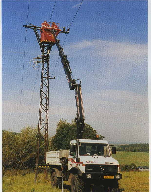
4-wheel drive trucks with radio-controlled Hiab cranes ensure power supplies to over 650,000 people in the central Czech Republic.
