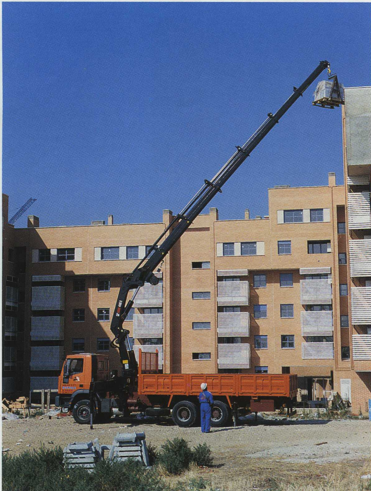
Masses of bricks are needed, and they are delivered directly from the brickworks to the building sites. A number of the brick works have obtained their own Hiab cranes so they can deliver the bricks precisely where they will be used.
