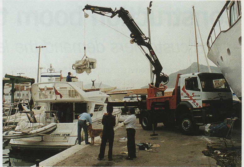
The engine weighs 1.6 tonnes and there are two centimetres to spare. A winch-equipped HIAB 245 E and CombiDrive radio control make this just another routine job for José Sarriá Núñez.
