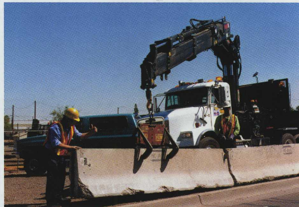
A HIAB 520-5, a grapple tool and CombiDrive radio control make light work of slotting in heavy concrete barrier walls.
