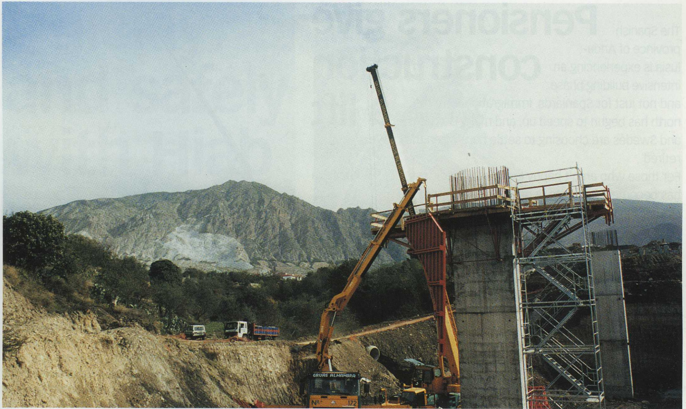
To speed up travelling time from Granada to the coast, a new motorway is being built the entire distance under the foothills of the Sierra Nevada. "This is just one of a number of bridges we're building," says operator Torcuato García Contreras of Gruas Alhambra S.L.
