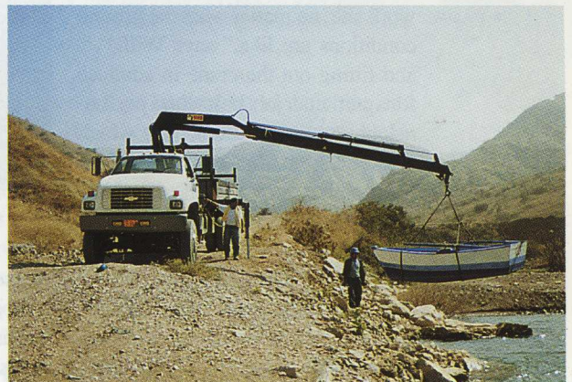
The Gallito Ciego building project, 4000 metres up among the peaks of the Andes, will boost Peru's power supply.
