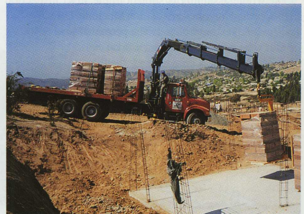
Brick deliveries with the help of pallet fork are easy and fast with the help of this HIAB 250-4 mounted on an International 4700.
