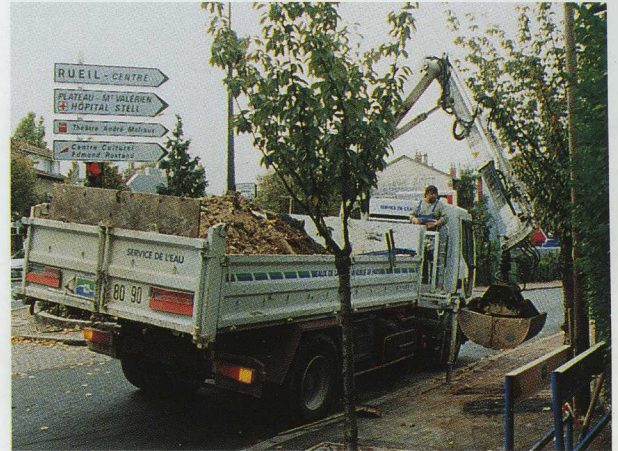
The pipe has been fixed and, with the help of his HIAB 090 AW and asphalt on his platform, Joël Trigueros sees to it that the pavement is as good as new.
