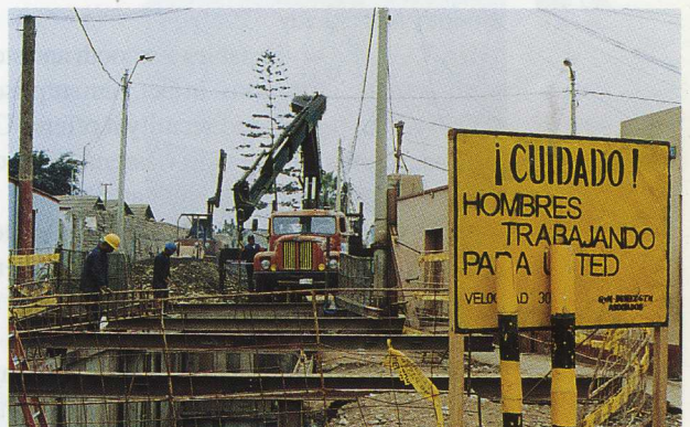
HIAB cranes being put to good use installing pipes in Lima's sewage system.
