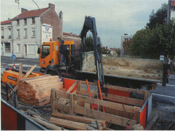
Some areas of the Paris suburbs are fairly hilly. "So we sometimes have to dig eleven metres deep to reach the main sewer which we are to connect a new pipe to," says Pires Manuel Leit ad. "I can reach down to four-and-a-half metres, after which a special excavator has to take over."
