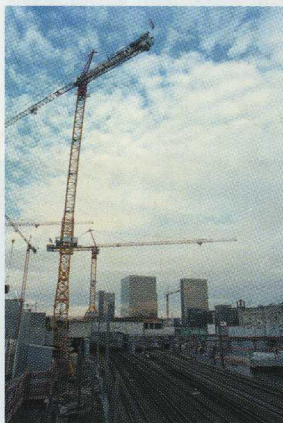
The Porte d'Ivry station by the Boulevard Masséa in Paris is one big building site.
