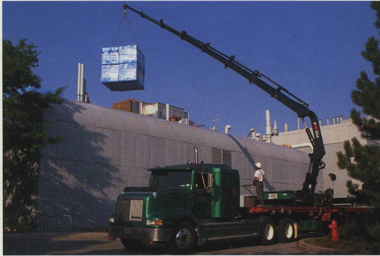
With the HIAB 225 E, placing the material exactly where Exeltherm's customers want it is a piece of cake for Robby Delorme.
