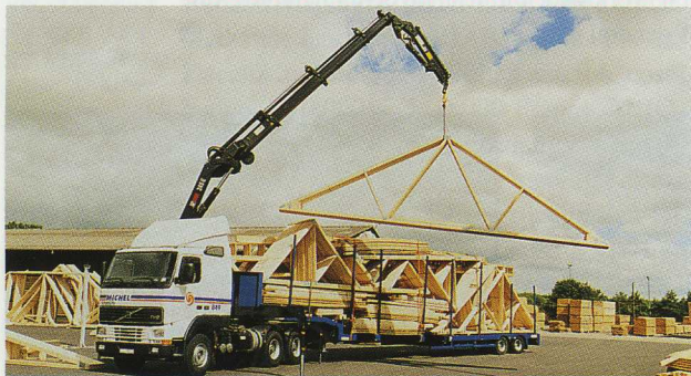
Long reach and optimum lifting capacity in all situations are important qualities for Transport Michel.
