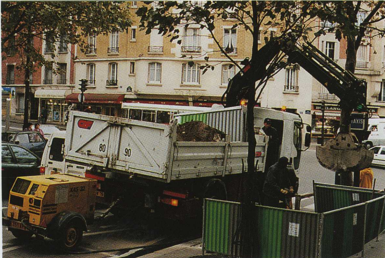
The little platform gives a clear view and helps the operator distribute the gravel and stones evenly. "We do this kind of work every day," says Jean-Luc Prevost. "...we get the foundations ready, JC Decaux deliver the bus shelter, which we then erect."
