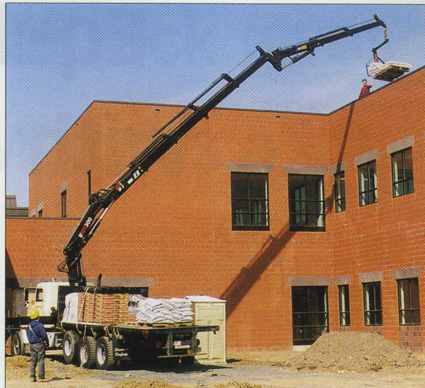
It is easy for Standard Roofing's truck to lift a pallet of roofing material into position with the help of its HIAB 300-4, a jib and a pallet fork.
