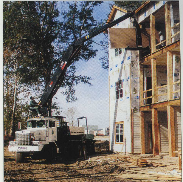
The special handling rig for wall units allows quick and efficient loading with the minimum amount of effort from building workers.
