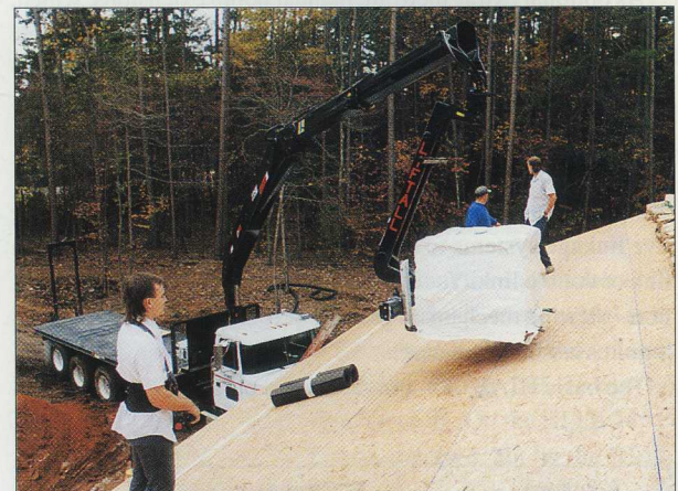
With the pallet fork it is easy to put roofing material down in the right place. Radio control of the crane allows the operator to choose the best position to work from.
