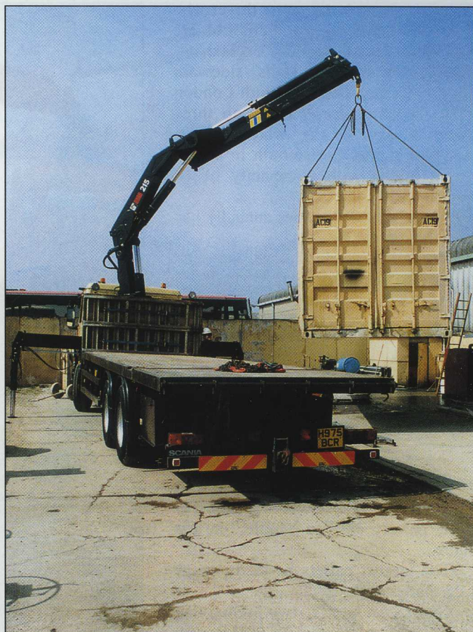
The new fireproof cabins demanded a stronger crane. Now there's no problem, nor with containers like this, filled with building supplies.
