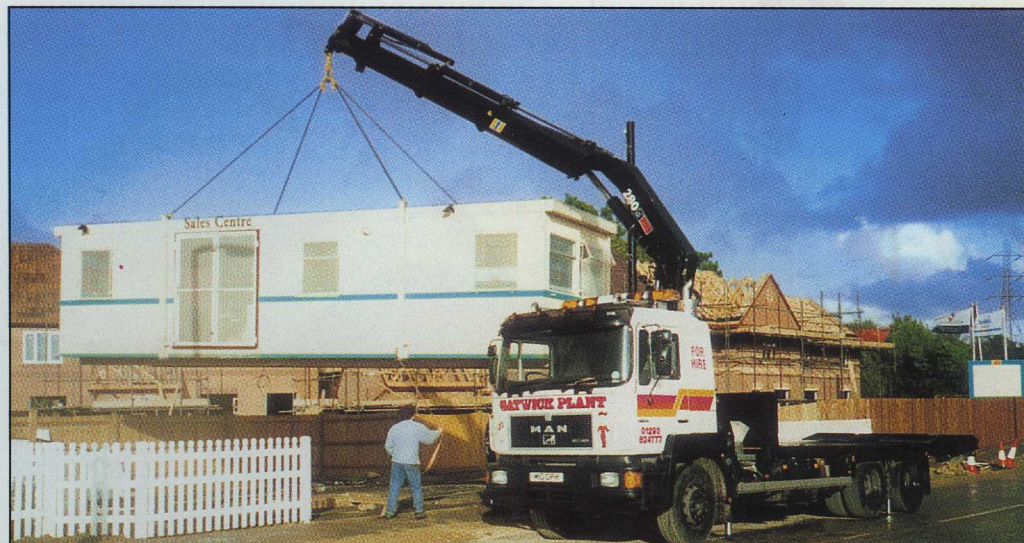
With HIAB CombiDrive these 4 tonne, 32 ft. (10 metres) cabins can be positioned with maximum safety.
