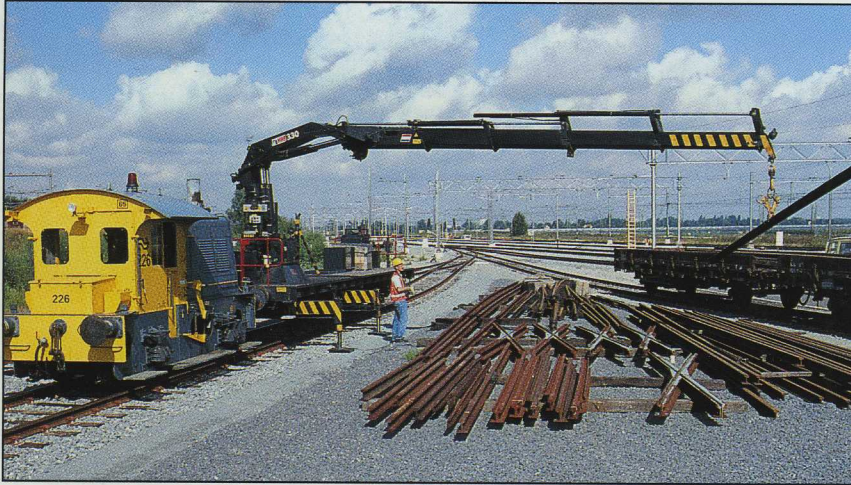
This HIAB 330-4 is used by Nederlandse Spoorwegen (NS), the Netherlands National Railway Company, to maintain and repair railway tracks in the Rotterdam area. It's equipped with a winch, HIAB CombiDrive remote control and HIAB SPACE Control. A short column was also specified so the crane could work inside Rotterdam's new Willems' Tunnel.
