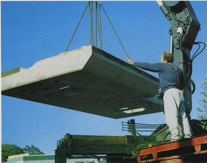
Gary Lane makes it look easy for one man to handle an eight tonne steel and concrete cover plate.
