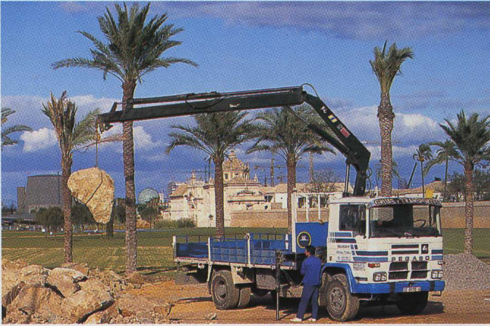
Silverio Ramirez (right), the owner of Silverio Transport S.L., has been in business in Seville for almost 18 years. He uses his HIAB 140 AW mounted on a two-axel Pegaso for loading and unloading a variety of building materials. One of Silverio's drivers (above) removing large boulders from a lawn. In the background are the monastery and ceramics factory which until recently were the only buildings on the Isla de la Cartuja, the site of EXPO '92.
