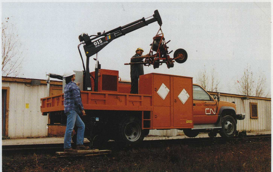
CN RAIL's Hy-Rail welder trucks are used for general maintenance work such as joining tracks and repairing switches.
