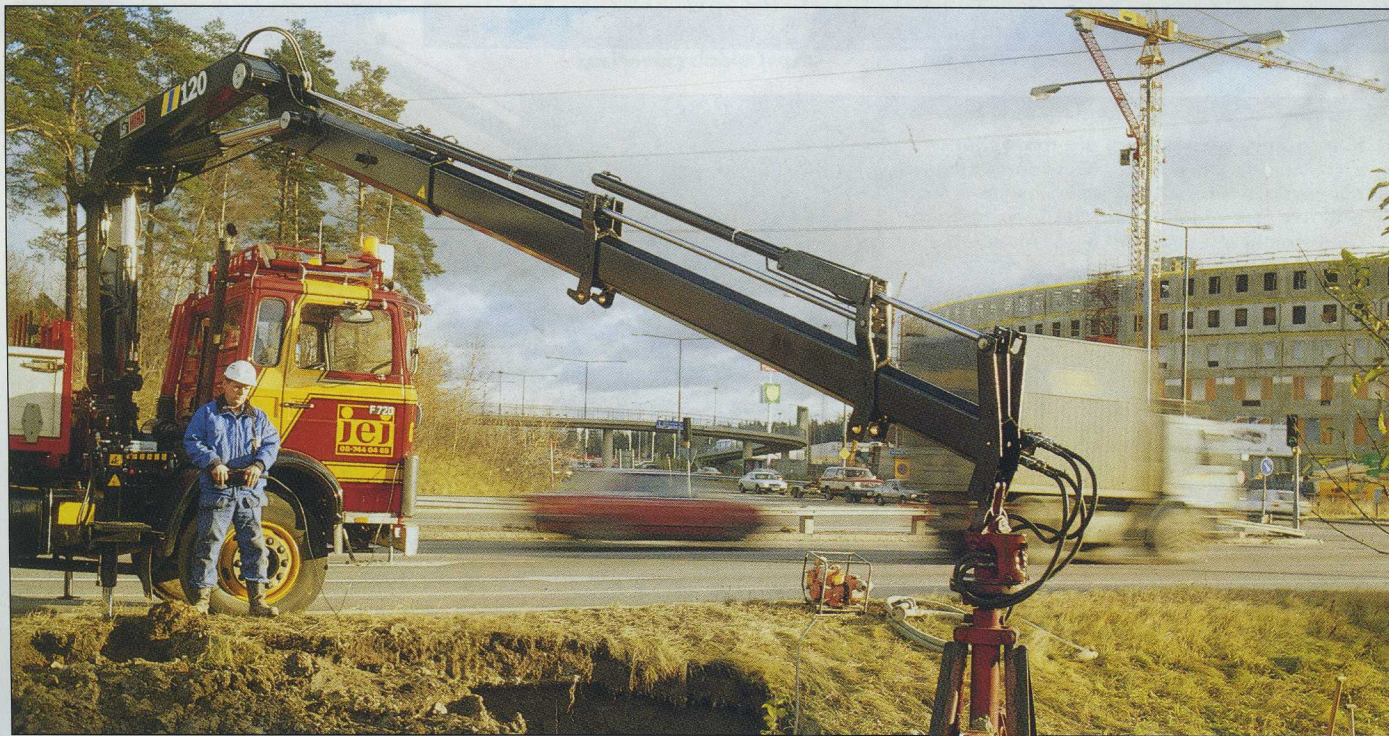
Equipped with a clamshell bucket, J. E. Jansson's HIAB 120 is used mostly for laying telephone cables.
