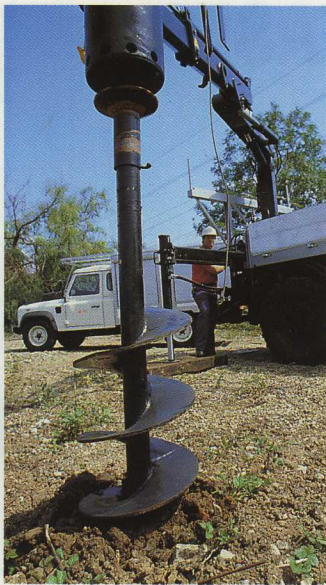
Eastern Electricity has several HIAB cranes fitted with earth augers that are used for boring holes and installing poles.
