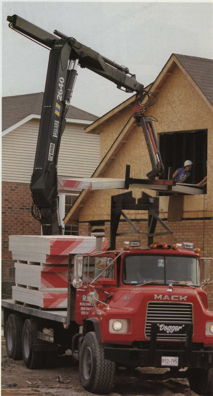
Russo Building Supplies located in Oshawa, Ontario, the centre of one of the highest growth areas of subdivision housing in Canada has a fleet of three HIAB 190s and a new HIAB 2640 that are all used to deliver drywall.
