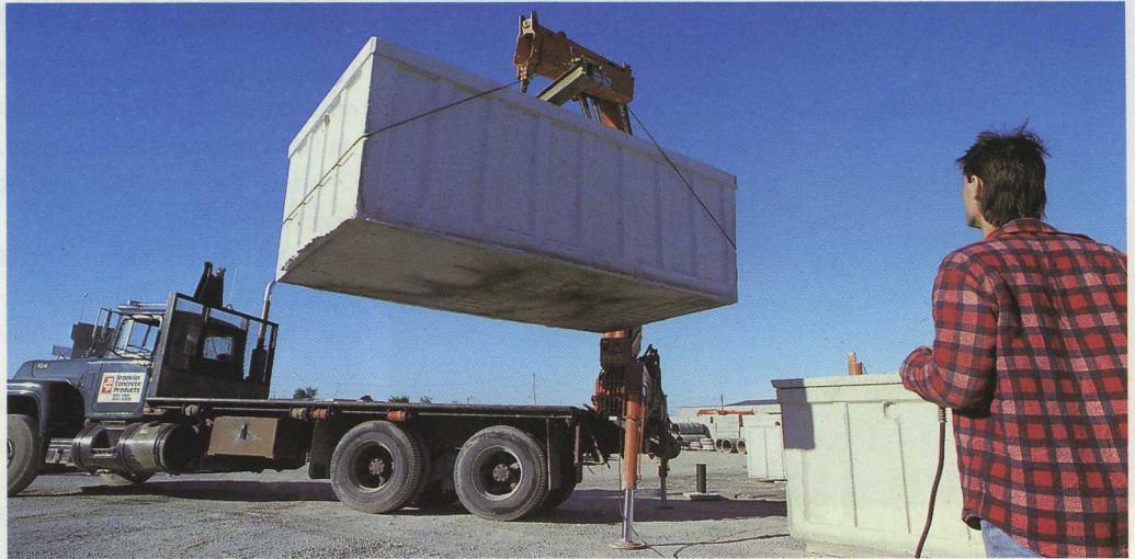
To place septic tanks accurately Brooklin Concrete Products Ltd uses a HIAB 260 equipped with remote control.
