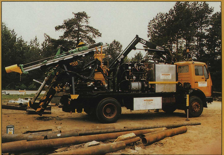
Talk about a well-equipped outfit! Two drill rigs. Vacuum cleaner. Compressor. And of course a HIAB 070 – with a "wrist" to make it even more manœuvrable.
