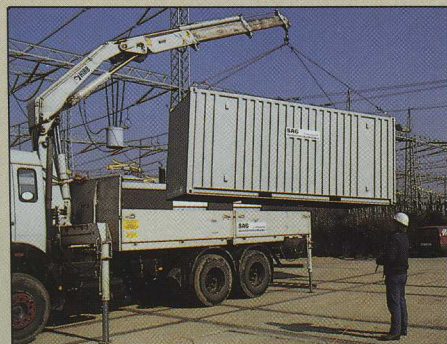
At this large power station, SAG has a DigiDrive-equipped HIAB 2070, a crane for heavy lifts.
