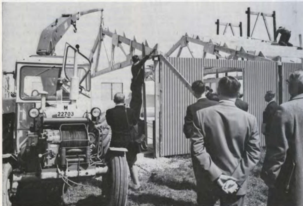
The prefabricated building was first put on display at the MILA Exhibition in 1964, where it attracted well-deserved attention. This picture shows a roof truss being mounted in the steel anchorages.
