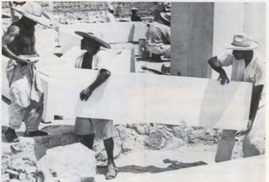
In many countries the supply of labour is seldom a problem, so that unloading a truck is often a wholly manual operation, as in this picture from Mexico. But truck time is always costly, so that the HIAB Method is beginning to gain a footing even there.
