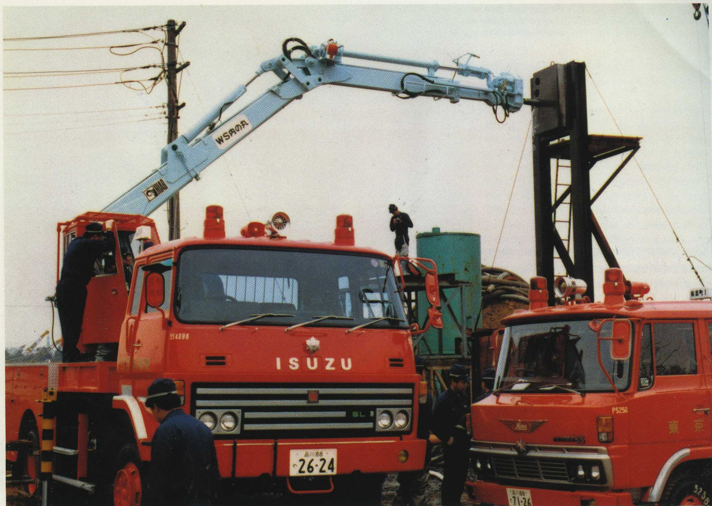
Here is the Tokyo Fire Defence Board demonstrating how to fight an inaccessible blaze by the HIAB Method. The cab enables the crane operator to get closer to the fire.
