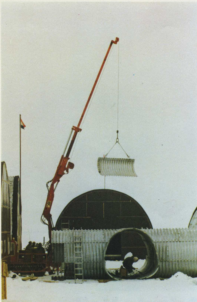
The buildings and communicating corridors of the camp are constructed from steel plates put into position by the HIAB 850s.
