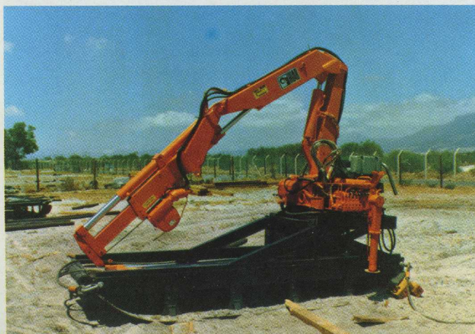
The problem of releasing the crawler while the loader was on stationary work was solved by the Method experts with a sled.
