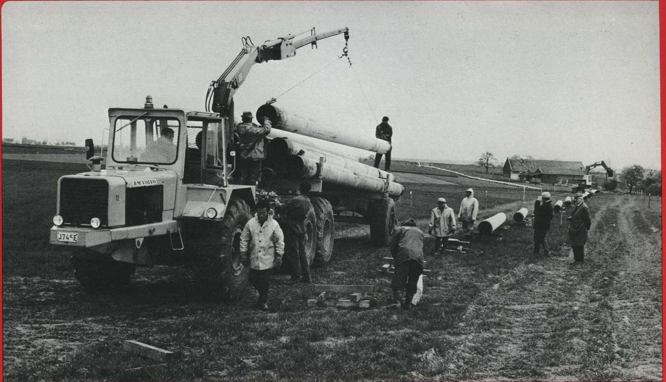
The trailer has a big payload and can quickly bring up large quantities of pipe.
