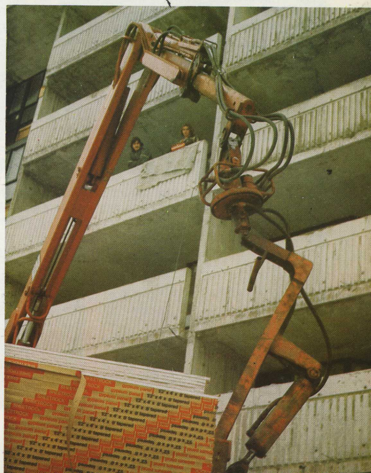
The hydraulically operated wallboard fork has returned to the truck to pick up a new bundle. The operator remains where he is on the balcony.
