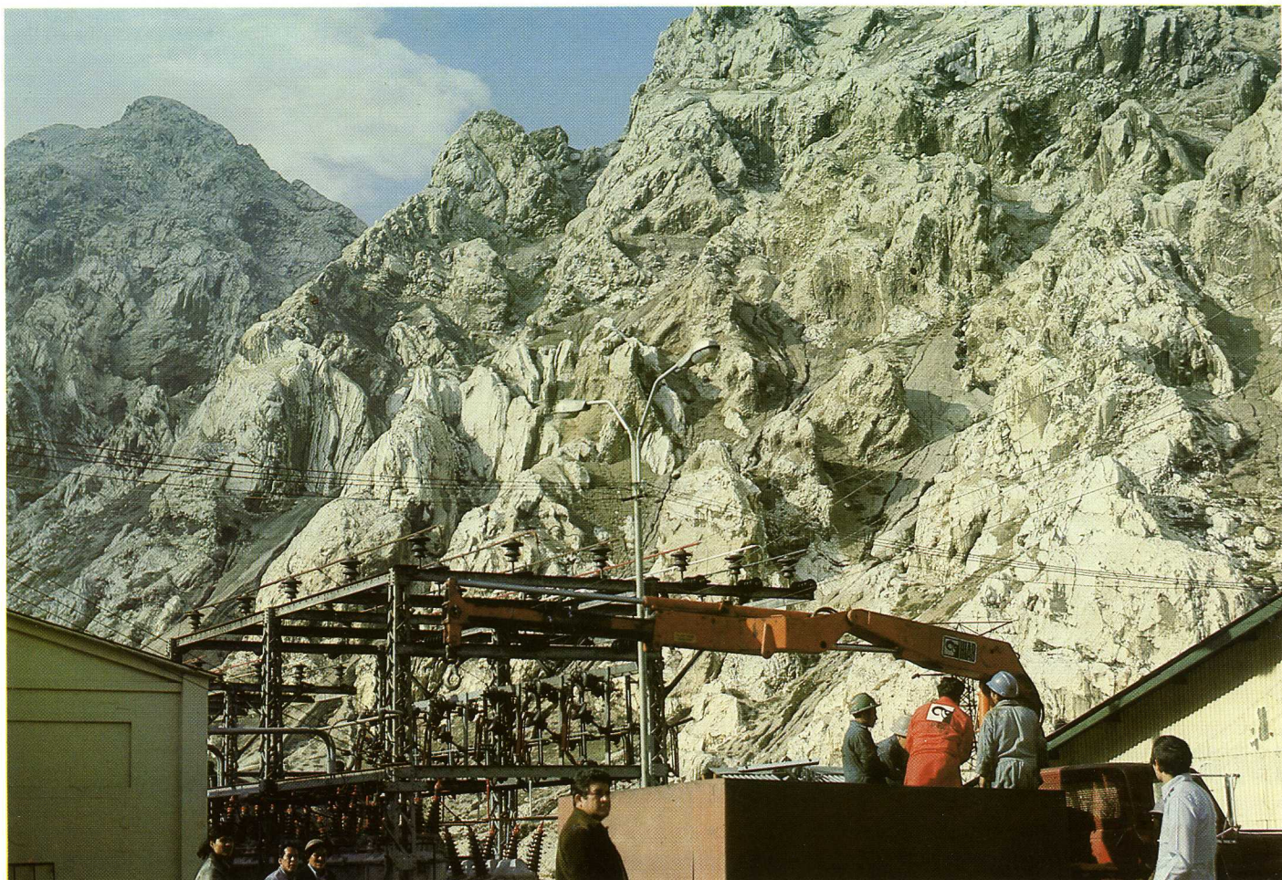
This loader works nearly 5,000 metres up at the hydroelectric power station of La Oroya, with the mighty peaks of the Andes forming the backdrop.
