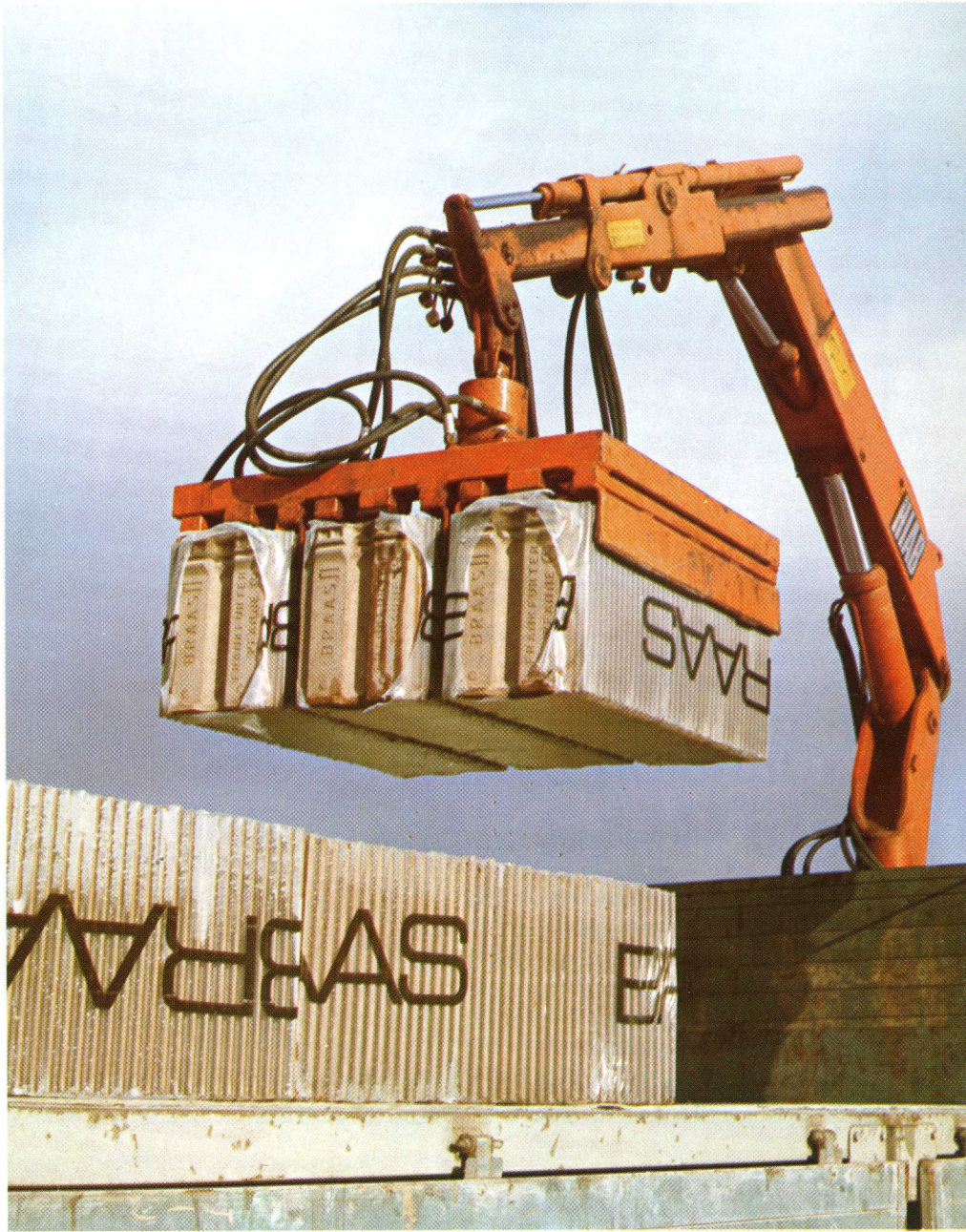
The grab can take both packed and unpacked tiles. This load is being delivered in 1-metre-long shrink-foil packs.
