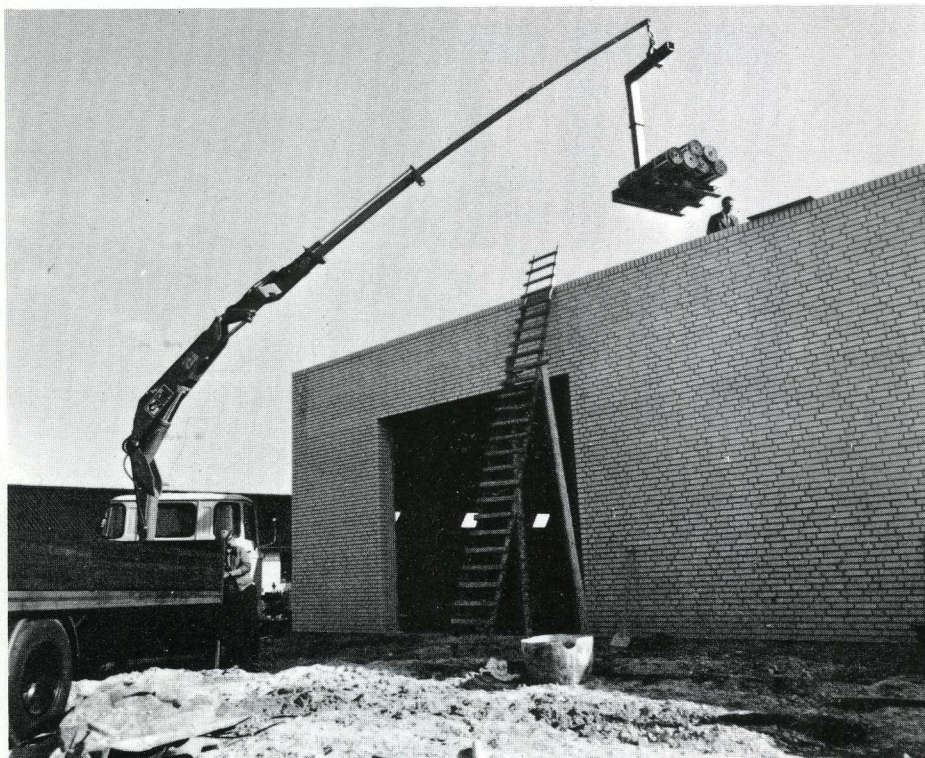
With two extra boom extensions the reach can be almost doubled to 9 metres and the roofing felt can be offloaded directly onto the roof.
