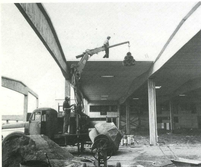
Karl Ludvigsson's old rig, equipped with a HIAB 550, is working on the same site, and is here seen lifting a load of roofing felt.
