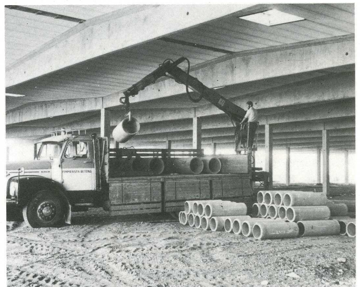
A load of concrete pipes at the site and is offloaded with the delivery truck's own HIAB. There is no building crane on the site.
