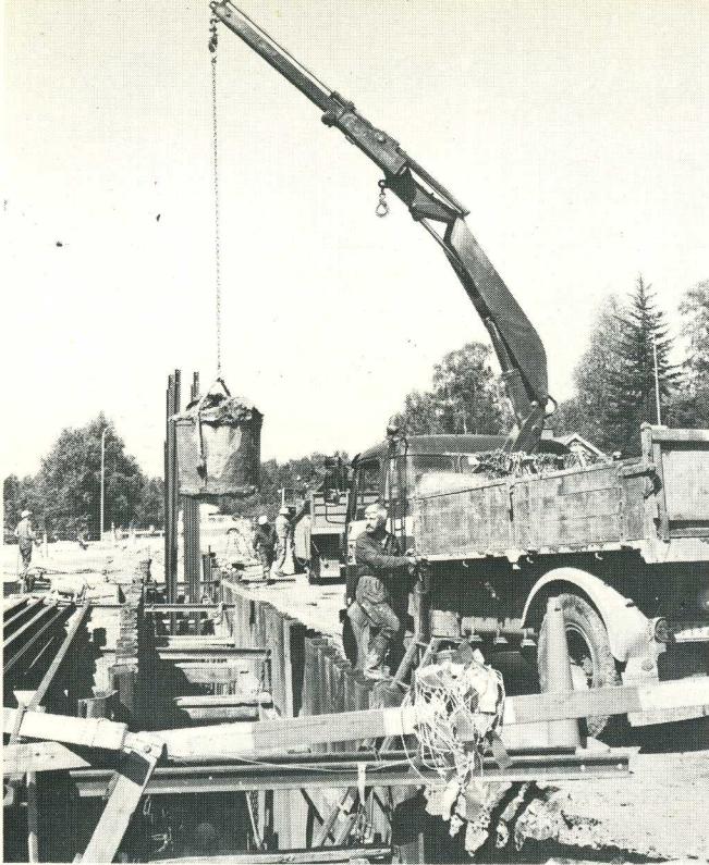
A fellow-trucker, also equipped with a HIAB 550, winches up the clay from the trench bottom.
