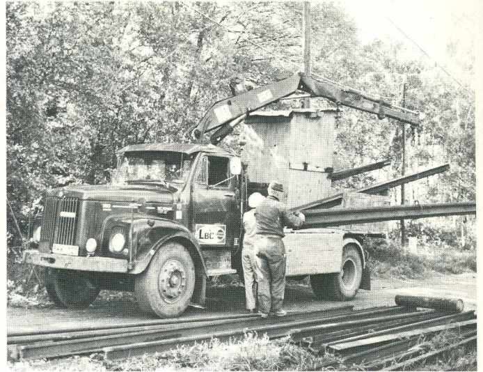
Next come some bundles of rails. Then it's the turn of the piledriver and the compressor. In this picture, piledriving is already under way.
