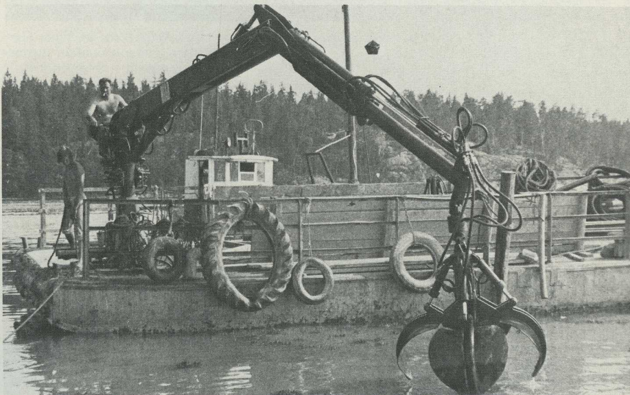
The old ferry draws only 60 cm and can move easily into shallow shore waters. Thanks to the great reach of the loader it can dig down to a depth of 3–4 metres. The dredging spoils are dumped on shore or into a 20-cu.-metre bin on the ferry.
