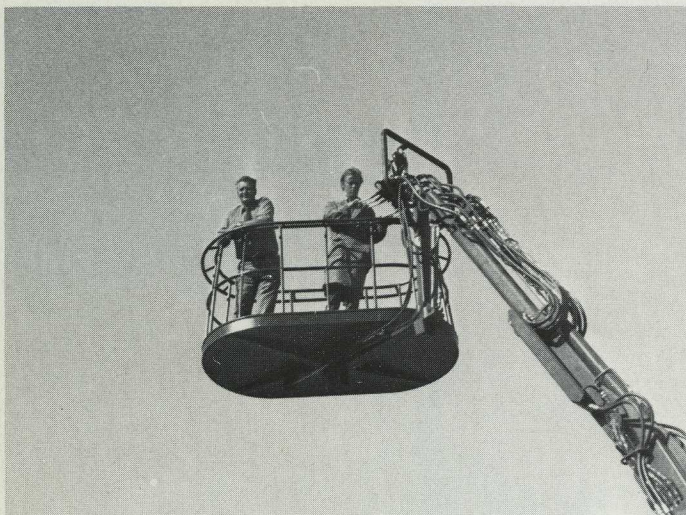
To give both the workmen in the basket the best possible position the platform is rotatable.
