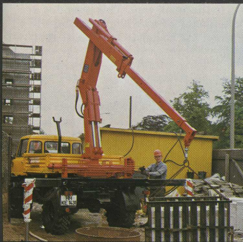
A pallet-load of building blocks is hooked up to the loader, and an instant later . . .
