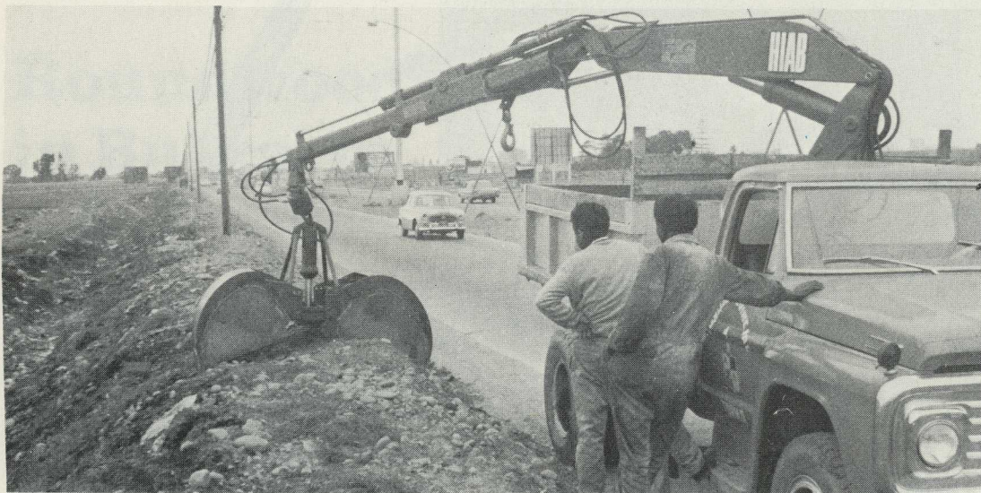
Here's the solution. A HIAB 550 with a clamshell bucket - an emergency substitute made from a round-wood grapple. It held the fort in fine style until a regular bucket arrived. An urgent order promptly dealt with!
