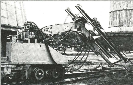
1 A jig with two hydraulic drills has been mounted on the outer boom, enabling the drill steels to be lined up with hydraulic ease.
