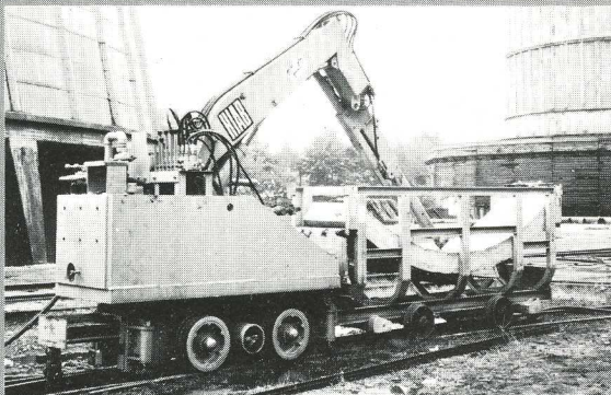
2 The concrete units are delivered to the point of installation in a transport car coupled to the loader car. Needless to say, they are loaded by the Hiab.
