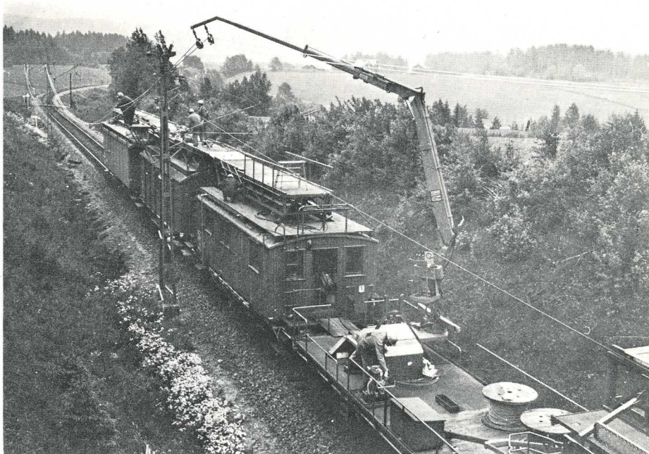
The Hiab Method provides the solution to one of the most ticklish problems in conductor changing: lifting the new conductors over the contact conductor and out onto the outside of the posts.
