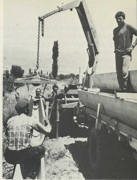
This is the way they install irrigation channels in Turkey nowadays. The Hiab Method has brought about substantial savings.
