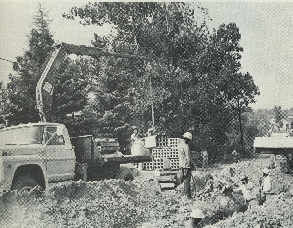
In the U.S. they put down sections of concrete conduits by the Hiab Method. The loader is remotely controlled, leaving the operator free both to hook on the conduit sections and then to walk over to the edge of the trench so as to get a good view as the section is lowered into place.
