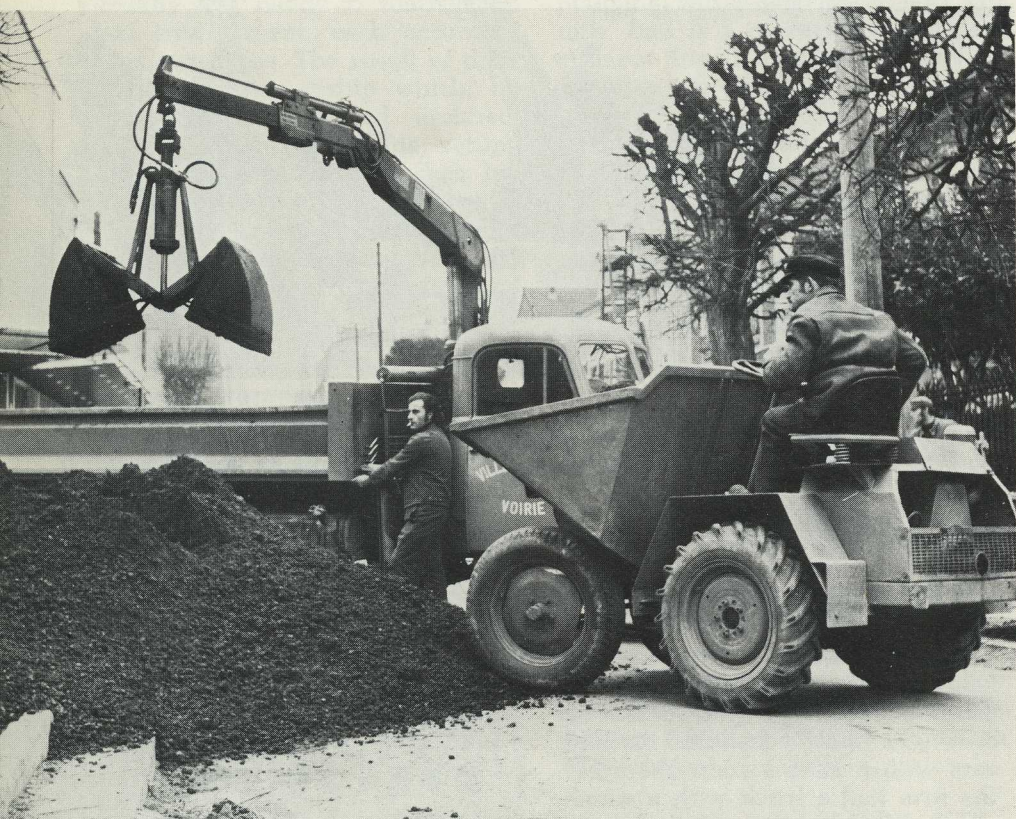
There's no mistaking how pleased the municipal workmen are with their Hiab Loader. Without it they'd have had a lot of spadework to sweat through here.
