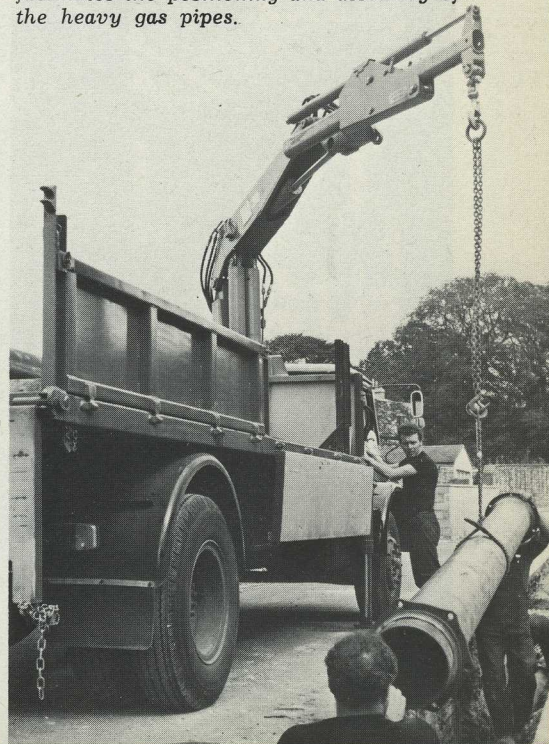
Precision handling with the HIAB 950 facilitates the positioning and assembly of the heavy gas pipes.
