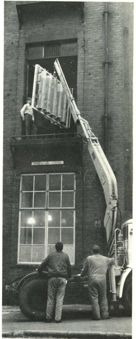
The HIAB 174 carefully hoists the wiring rack of a telephone exchange directly to the place on the first floor where the exchange is to be installed.
