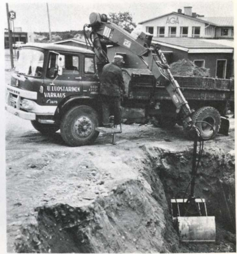
Trucker Urho Luostarinen of Varkaus has a HIAB 174 equipped with a 1000-kg hydraulic winch plus a clamshell bucket with a rotator. The outfit is employed on municipal works, excavating trenches, laying water mains and sewers, and transporting gravel.
