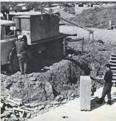
Down on the foundation slab the future householder takes delivery in person.
