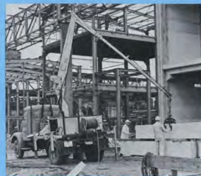
At the rear of the rig is a platform onto which the whole parcel of concrete units can be loaded.
