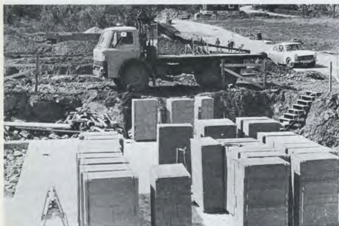
The entire load has here been lifted by the HIAB loader down onto the foundation slab and distributed evenly over the building area to ensure that the amount of movement during the actual erection will be at a minimum.
